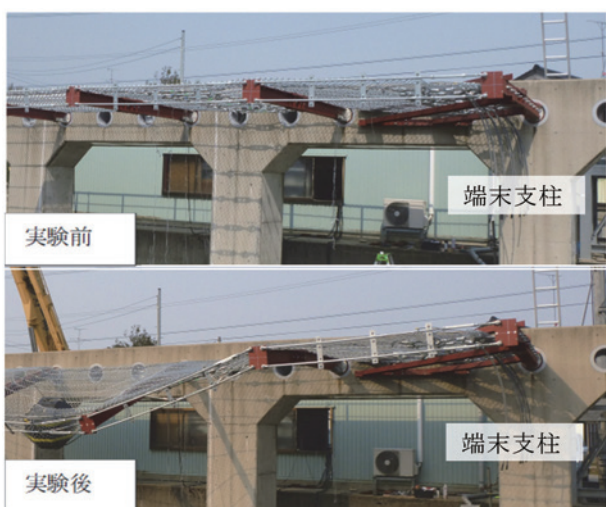
写真-11 端末支柱の変形状況 (CASE-3) Photo11 Deformation of terminal post
