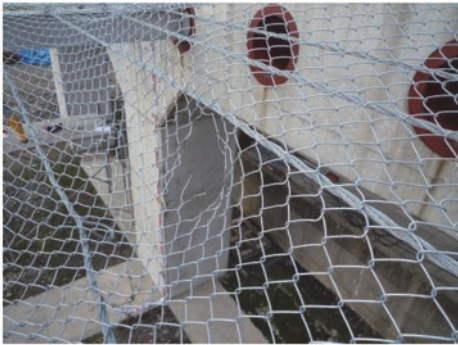
写真-6 金網の破れ (CASE-1) Photo 6 Breaking the wire mesh (CASE-1)
