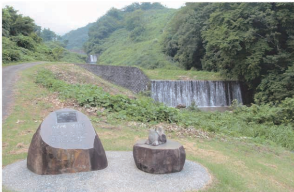
図一四 万内川一号堰堤 (1925 (大正 14) 年完成) Fig. 4 Bannai River No. 1 sabo dam (Completed in 1925)
